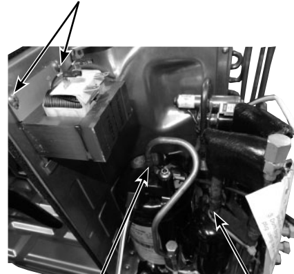
Discharge pipe brazed part
